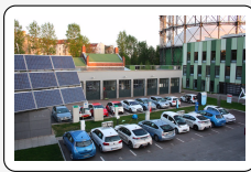
EV charging station
